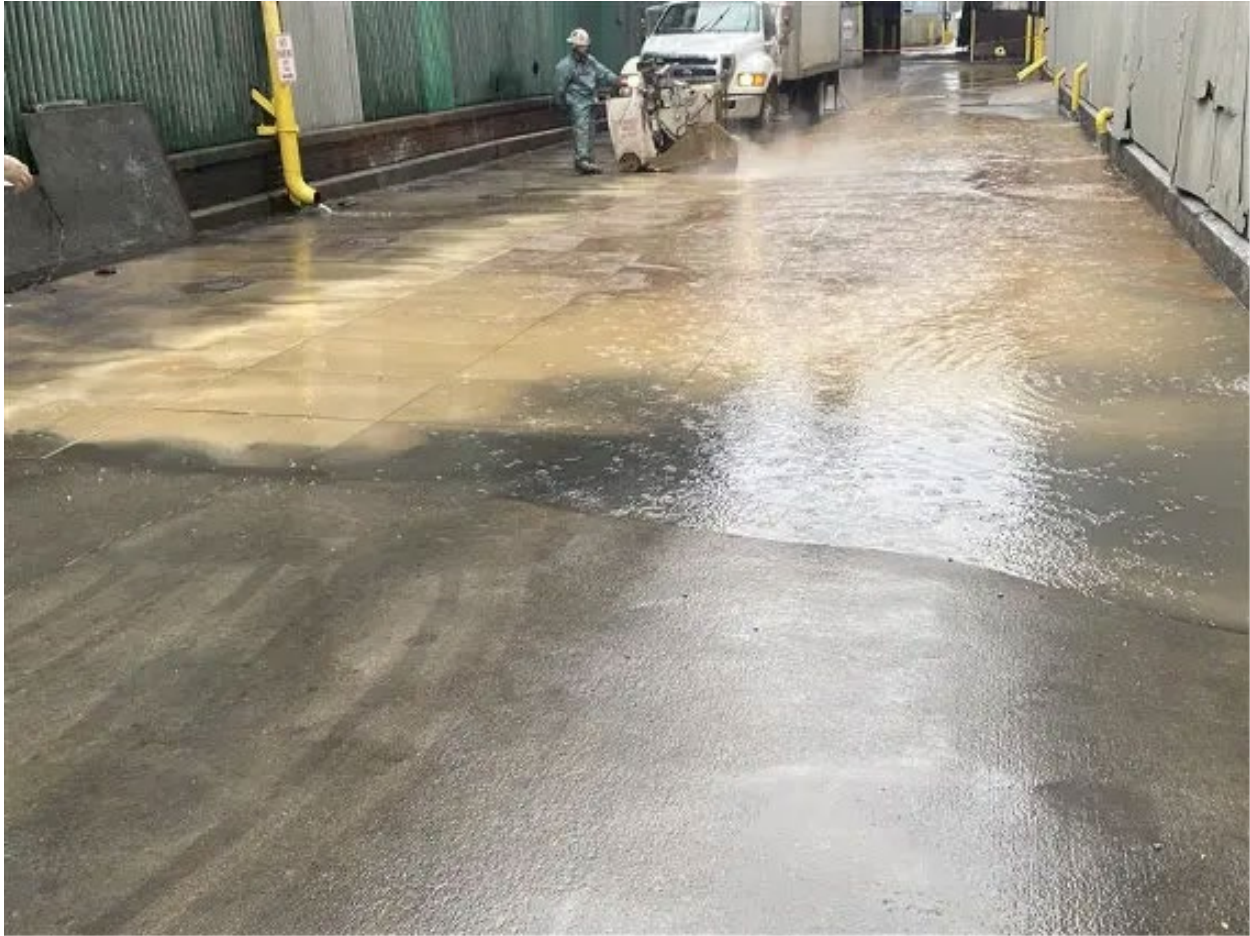
Image Description: Flooded job site due to massive underground water leak at plant
