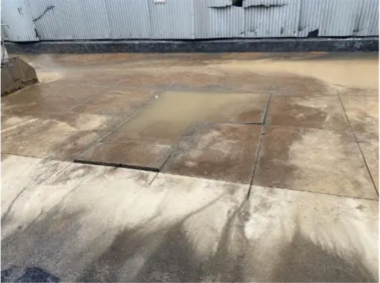
Image Description: Concrete slab sinks into the ground once saw cutting occurs due to an 8" ductile iron water line with a full circular break.
